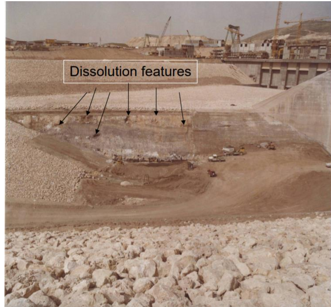
Figure 3: Photo taken during construction of Mosul Dam (1982-1983) historic dissolution of gypsum prior to dam construction. (Photo provided by A. T. Ayoub.)
