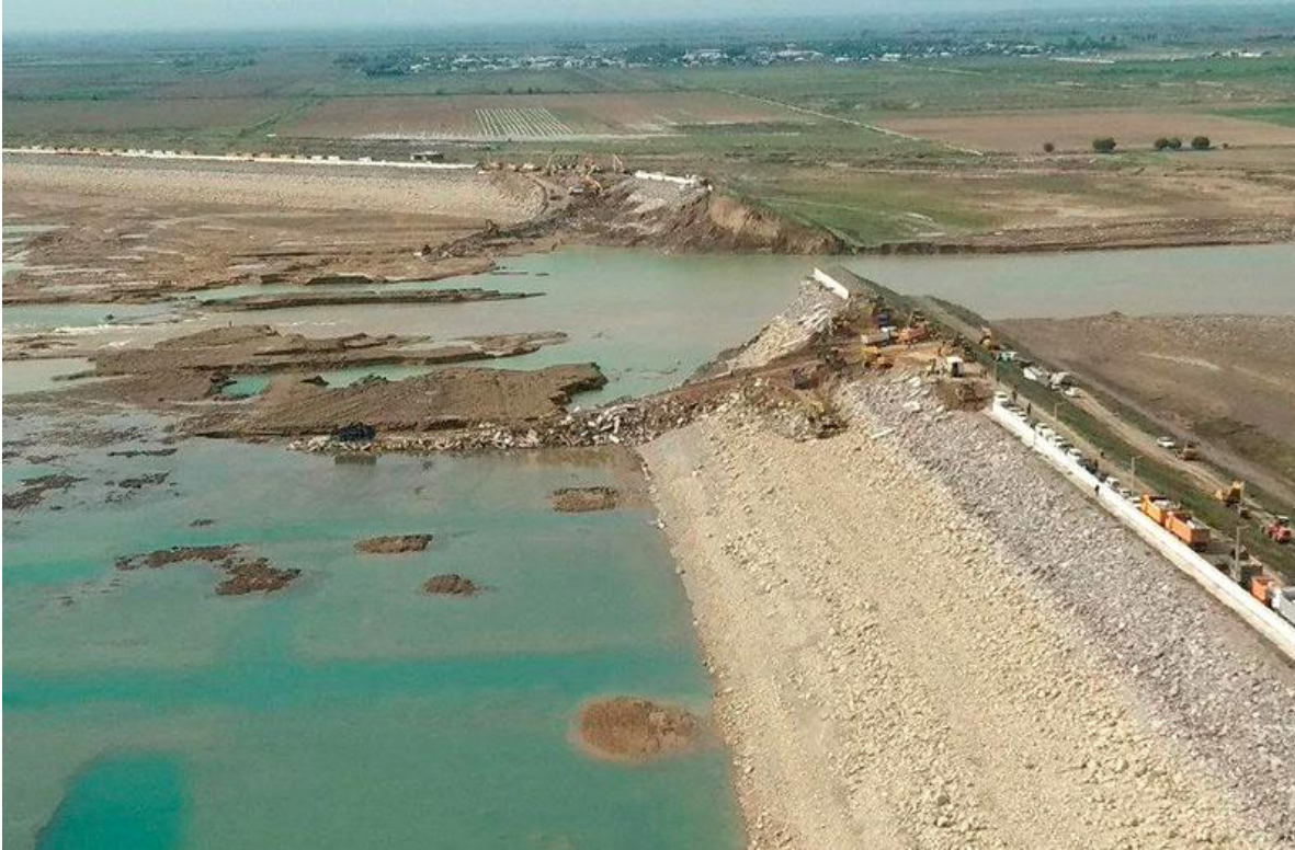
Sardoba Dam Failure (29 m), Uzbekistan (2017 – 2020)
